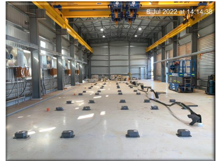
Power station gas engine shed
