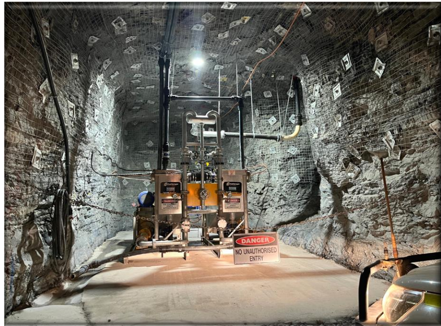
Underground pump station
