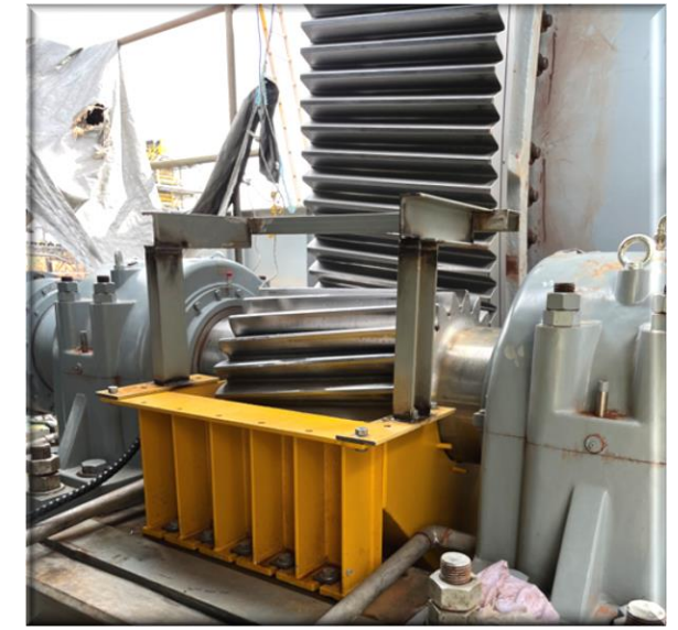
Mill Pinion & Girth Gear
