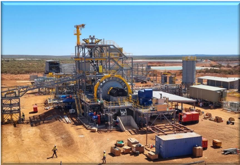
Grinding, Flotation & Filtering Sections
