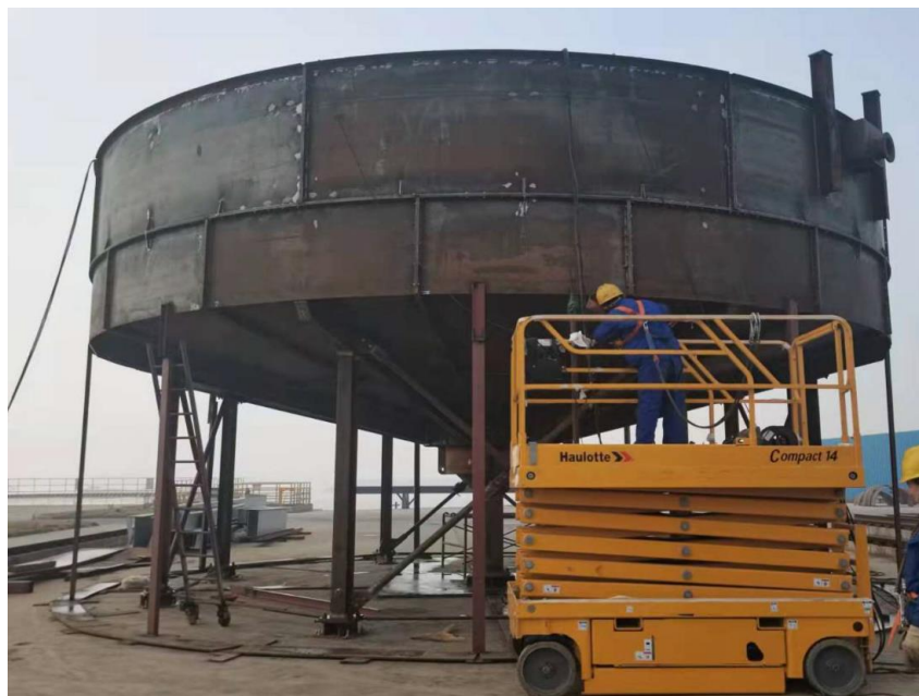
Figure 7. Processing Plant equipment fabrication (concentrate thickener).
