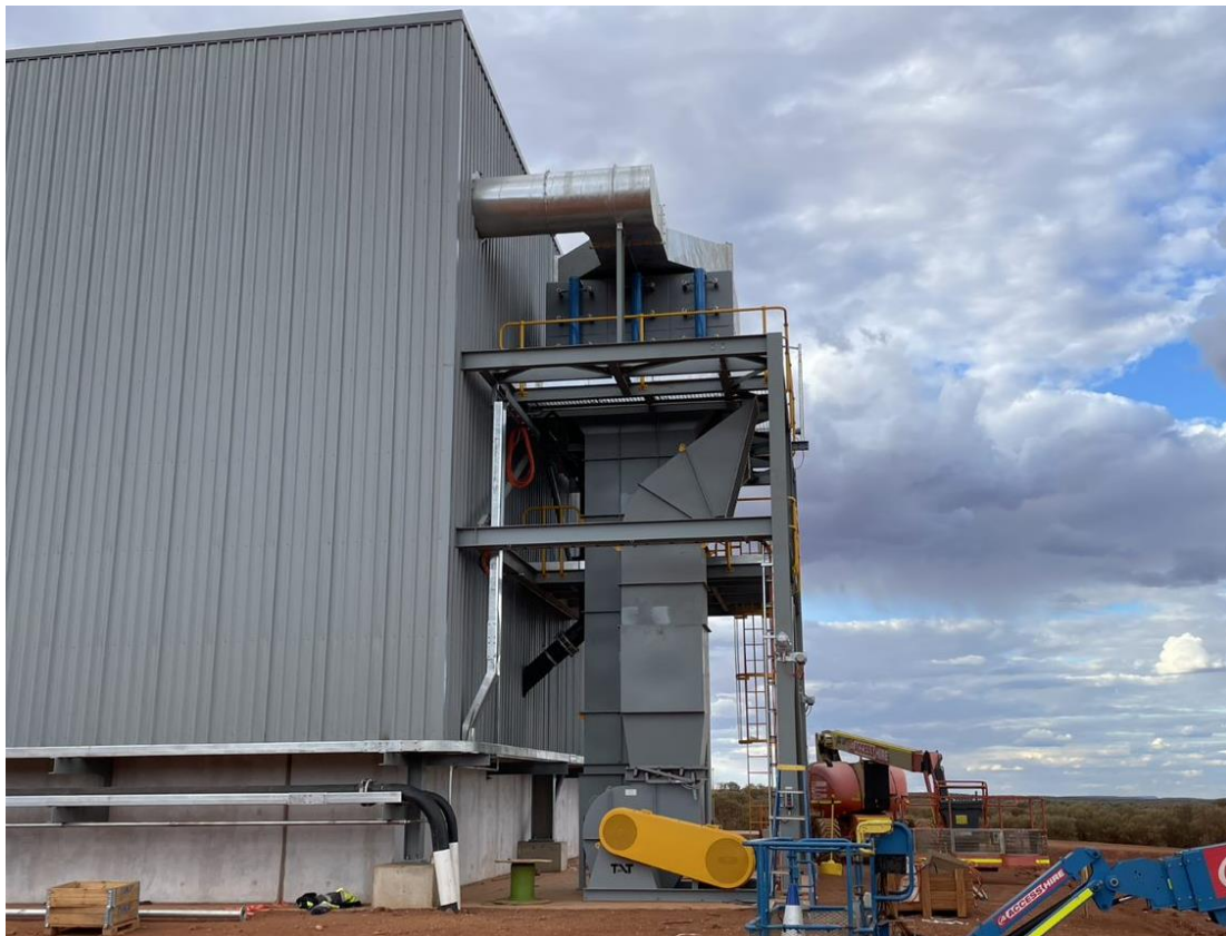
Figure 13 – Concentrate shed Dust Extractor.
